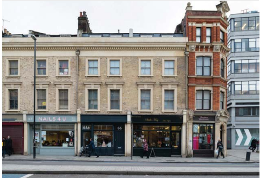
High Street 2012, London Borough of Tower Hamlets. Many historic buildings along the High Street 2012 route had fallen into a state of disrepair and had undergone unsympathetic modernisations. The Whitechapel phase of this initiative saw 61 properties restored to their former glory
