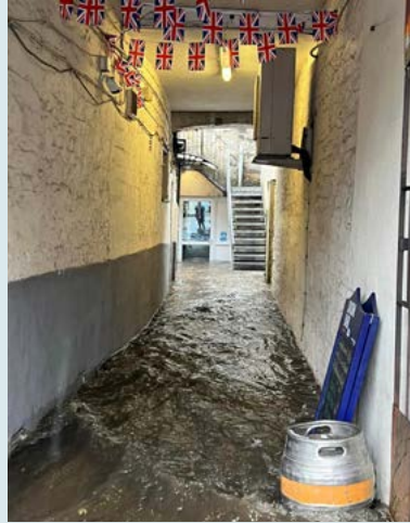
Flooding in June 2023
